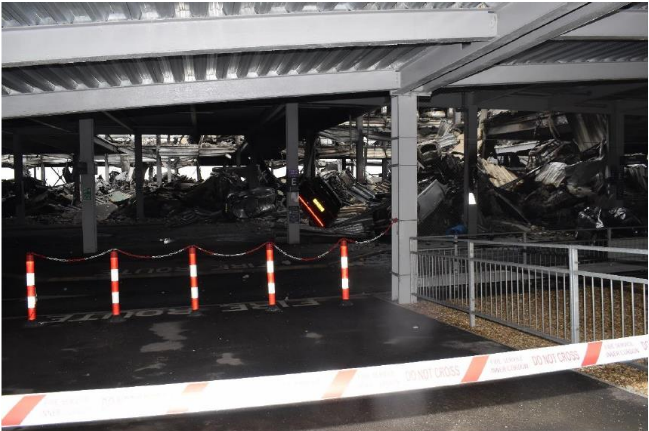
Figure 7 – Image showing building collapse post fire. Image is used courtesy of Bedfordshire Police
